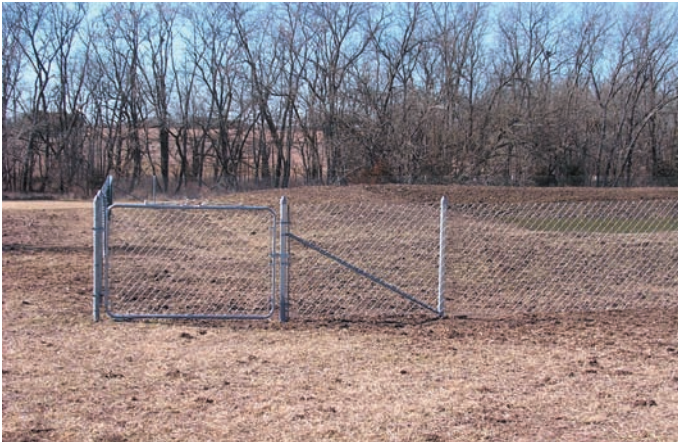
Figure 1. A lagoon with a good fence and gate outside toe of embankment.
